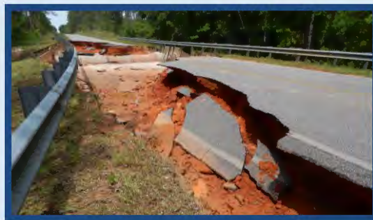
Flood damage in Perdido Beach, AL. Photo Credit: Patsy Parker, May 2014.
