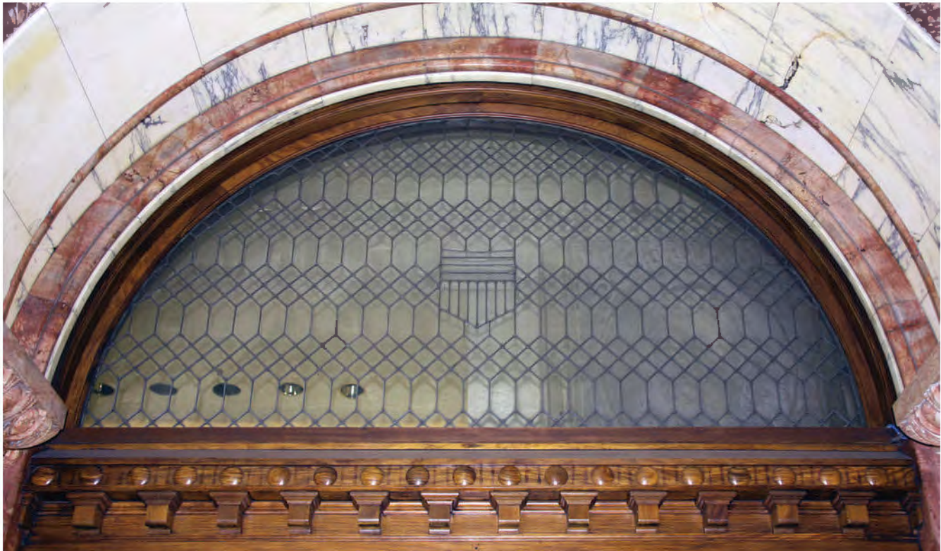
FIGURE 47: Detail of Tower Lobby Feature Wall Transom, 2012. Image Courtesy of OLBN Inc.
