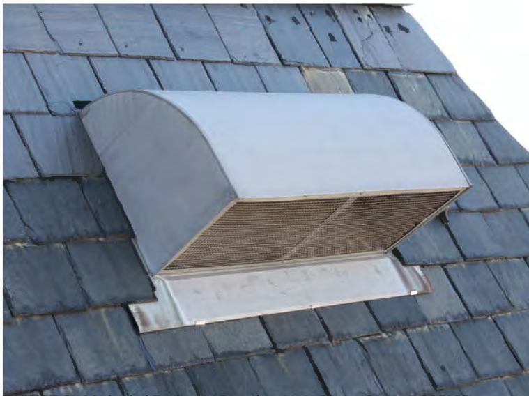
FIGURE 52: Mechanical Equipment Intrusion, 2012. Photo Courtesy OLBN Inc..
