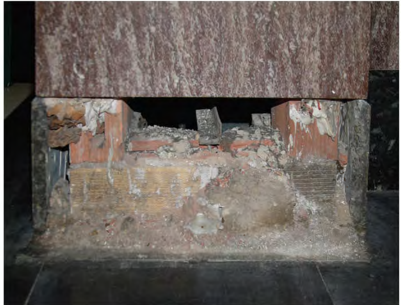
FIGURE 85: Missing Baseboard Slab, 2012. Photos Courtesy OLBN Inc.
