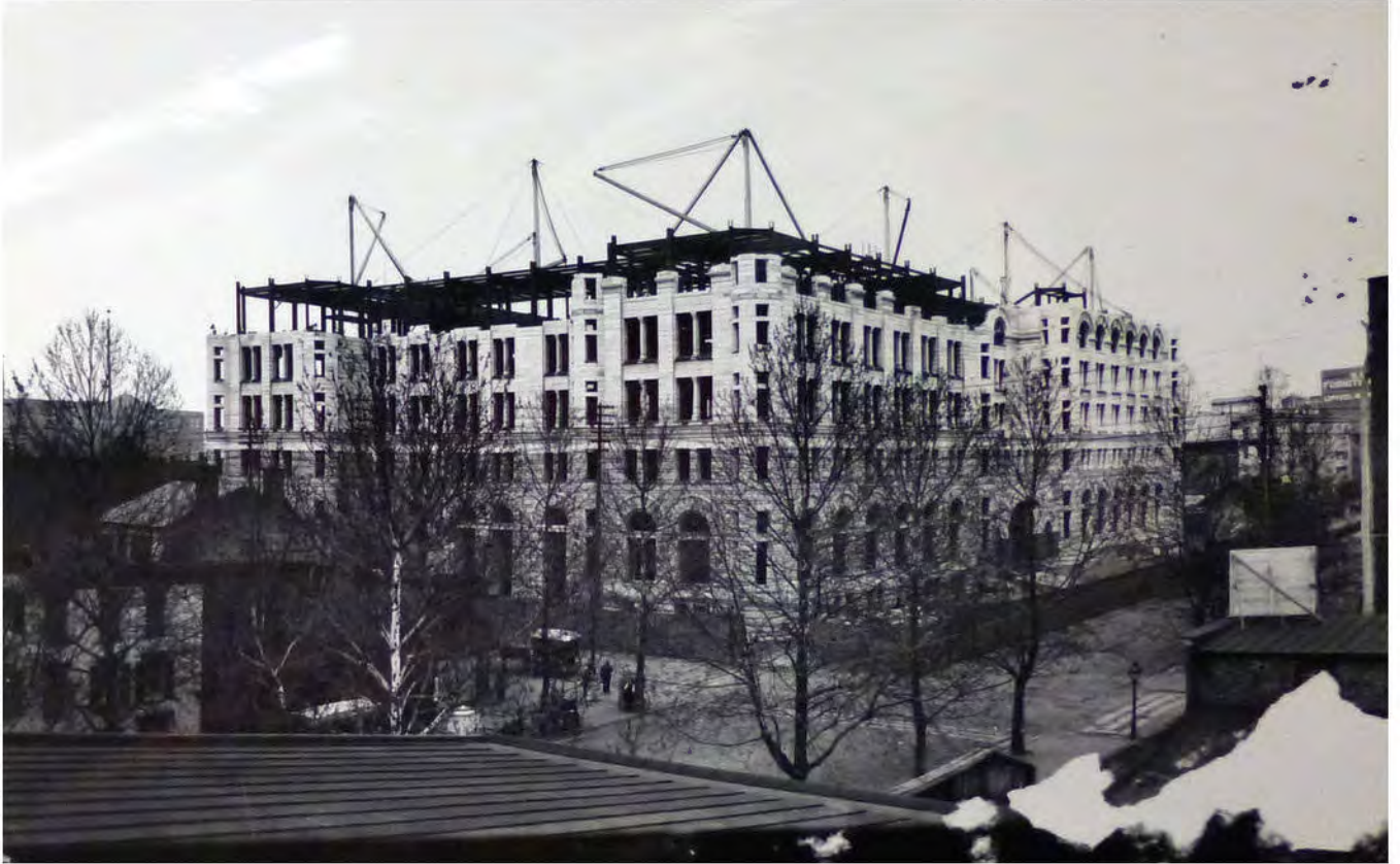
FIGURE 1: Post Office under construction; structural skeleton can be seen behind stone façade. Image Courtesy of the National Archives and Record Administration, Cartographic and Architectural Records, College Park, MD, Record Group 121
