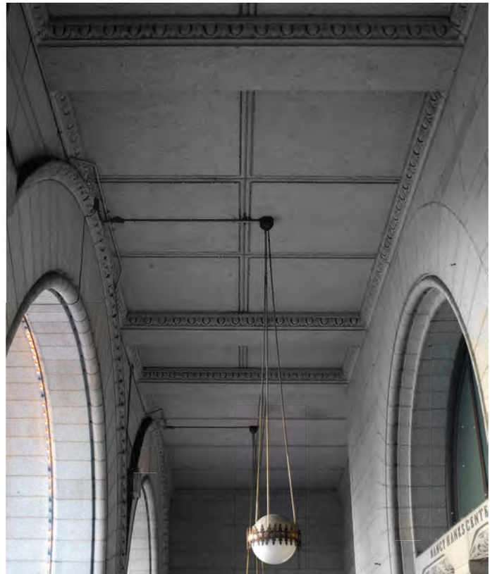
FIGURE 62: Pennsylvania Avenue Portico Ceiling, 2012. Photo Courtesy OLBN Inc.
