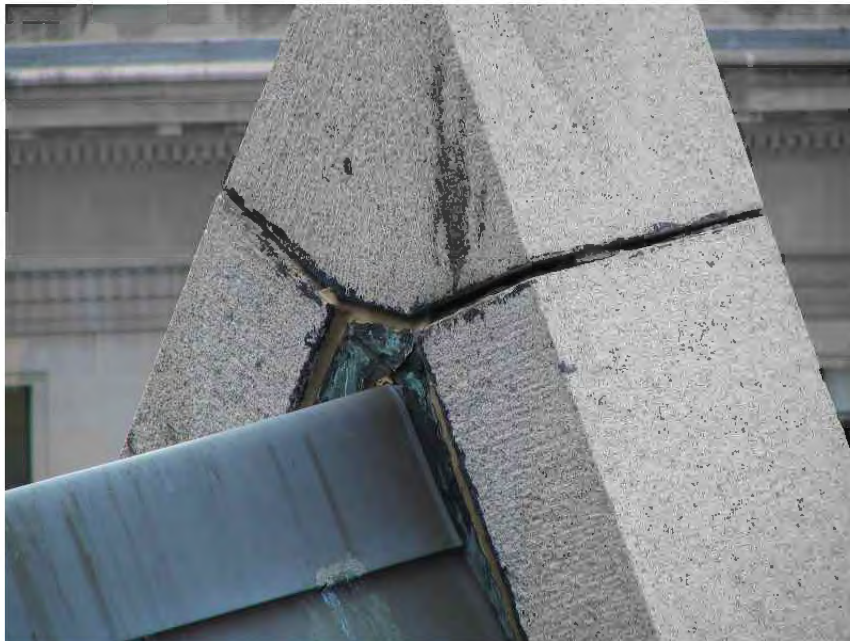
FIGURE 4: Dormer Parapet Wall With Open joints, 2006. Photo Courtesy of T. McDowell.
