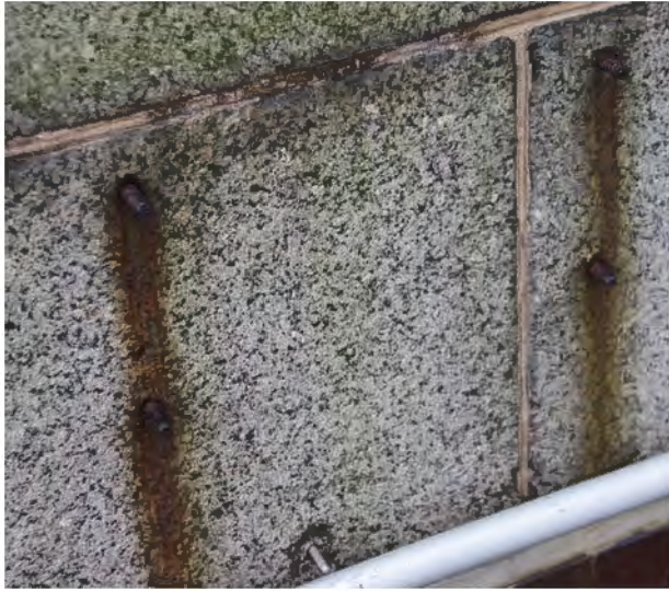
FIGURE 6: Pennsylvania Avenue West Wall Rust Staining, September 2012. Photo Courtesy OLBN Inc.
