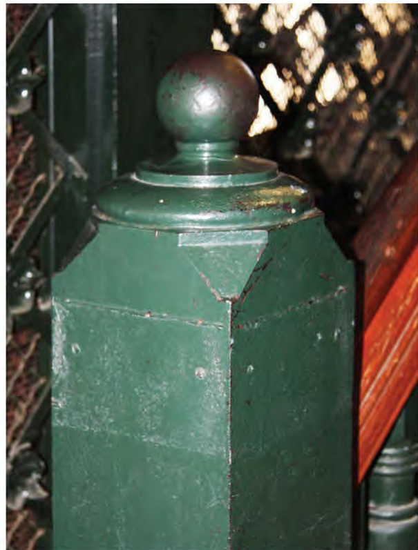
FIGURE 34: 12th Street 1st Floor Newel Post, 2012. The paint has chipped and the red lead primer coat is starting to show in some parts, in others it has rubbed off. Photo Courtesy OLBN Inc.
