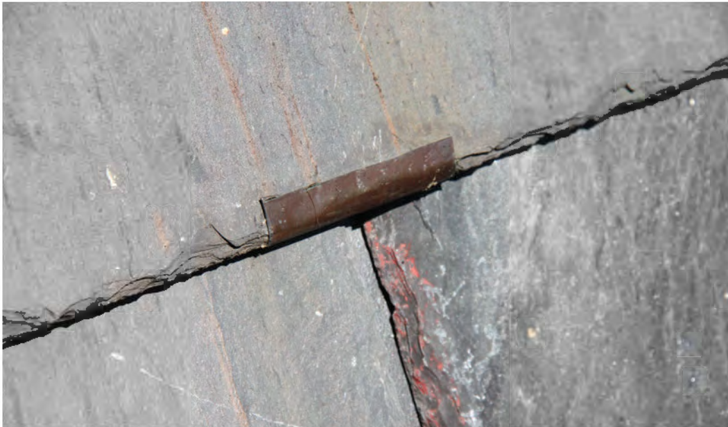
FIGURE 49: Shingle Installed Using A Sheet Metal Tab Turned Up Over The Bottom Edge Of The Shingle, 2012. This is a type of repair not recommended where snow and ice can cause the tab to straighten out so that the shingle slips out of position. Photo Courtesy OLBN Inc..
