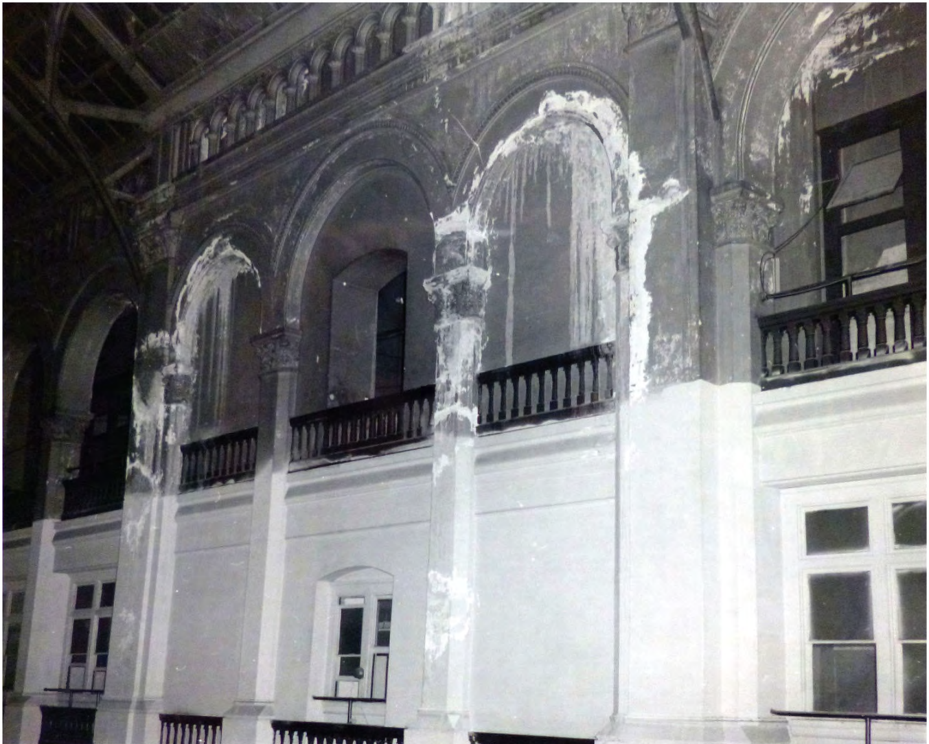
FIGURE 30: Undated photograph of cortile arcade, showing water damage. Image Courtesy of GSA-NCR Technical Resource Center, Reports and Photographs
