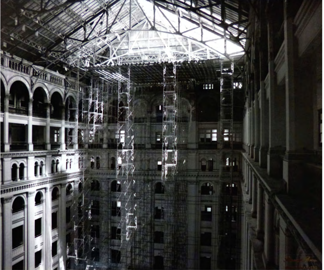
FIGURE 37: Construction progress photograph showing removal of roofing panels, 1979. Image Courtesy of GSA-NCR Technical Resource Center, Reports and Photographs
