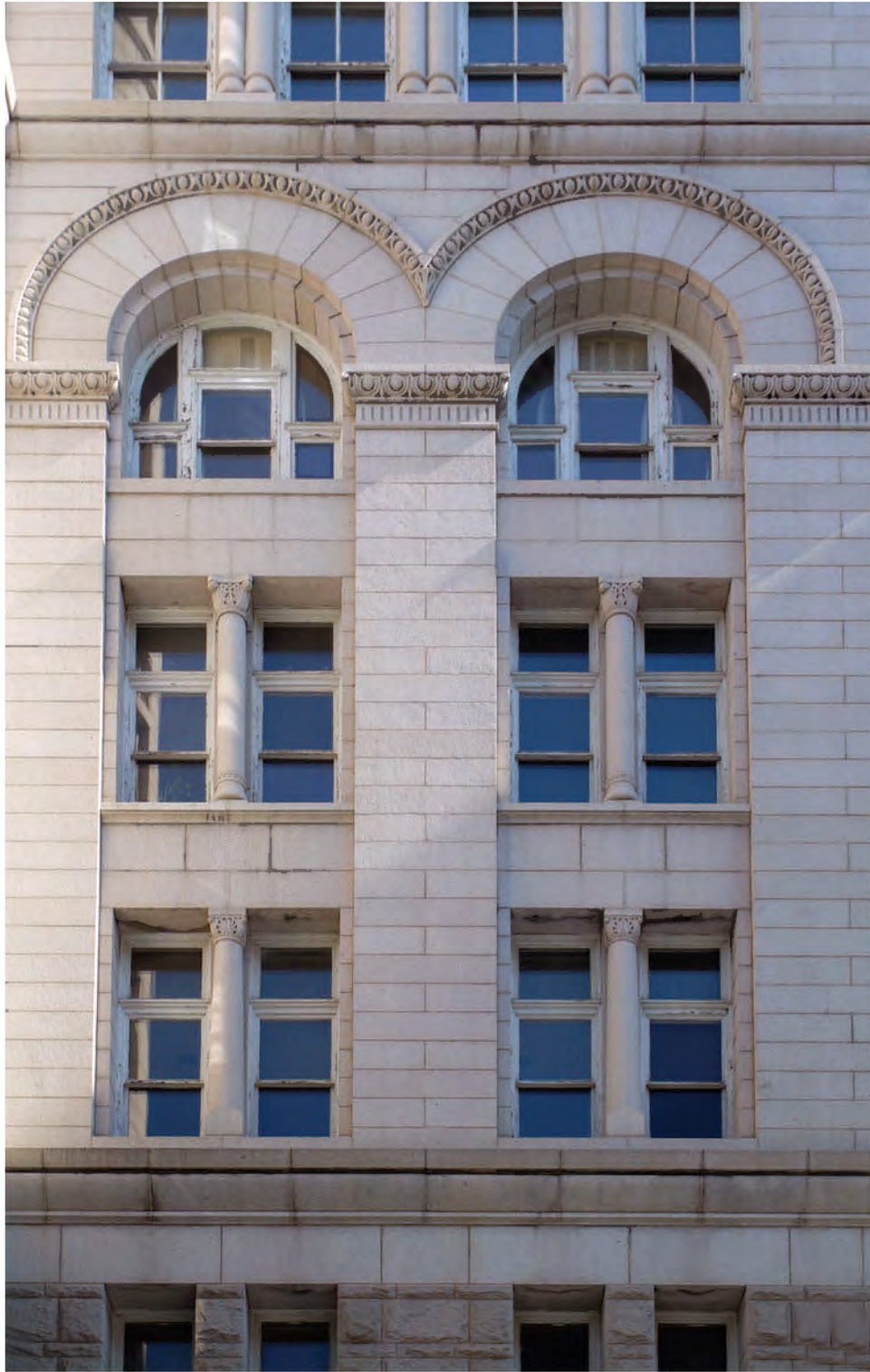
FIGURE 22: Detail of the NE Pavilion 3rd, 4th and 5th Floor Fenestration Openings, 2012. Photo Courtesy OLBN Inc.
