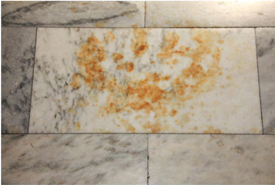
FIGURE 75: Rust Stains on the Corridor's Marble Floor, 2012. Photo Courtesy OLBN Inc..
