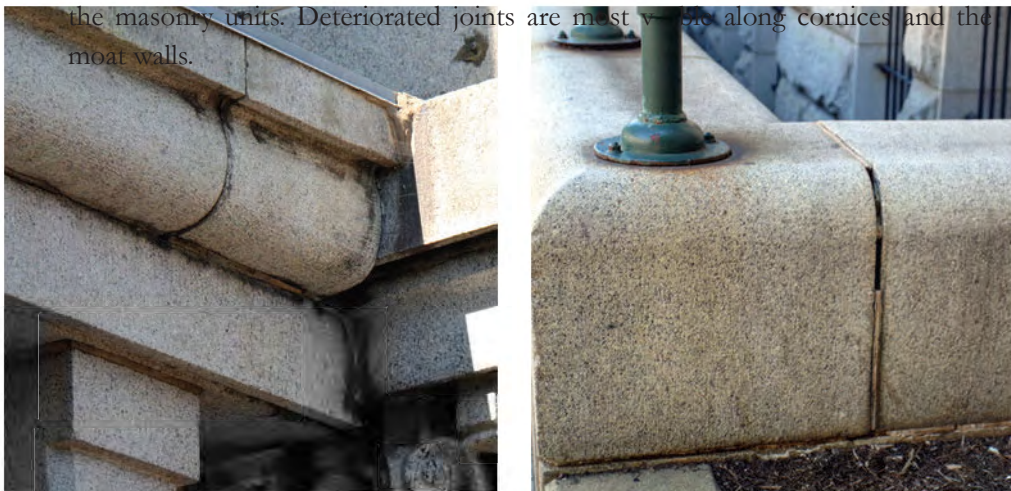
FIGURES 22 & 23: Missing and Eroded Mortar, 2012. Photos Courtesy OLBN Inc.
