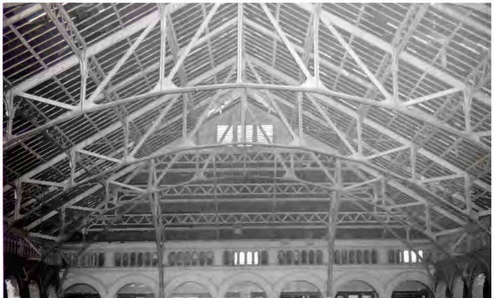
FIGURE 96: Photograph of the Skylight Over the Cortile of the Washington D.C. Post Office. Image Courtesy of GSA-NCR Technical Resource Center.
