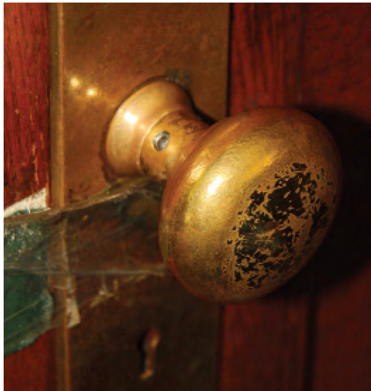
FIGURE 38: Interior Office Door Knob Showing Tarnish, and Overall Poor Condition, 2012. Photo Courtesy OLBN Inc.
