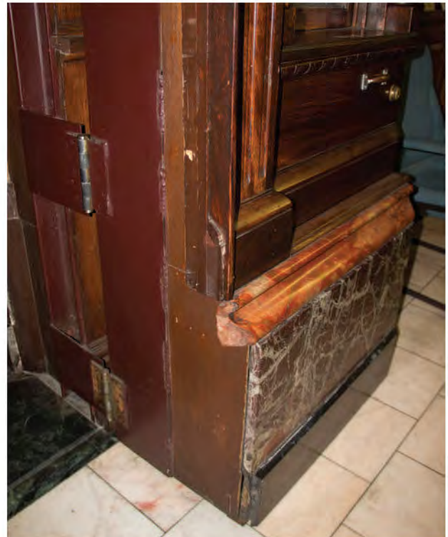
FIGURE 53: Detail of Tower Lobby Feature Wall Hidden Door Hardware, 2012. Image Courtesy of OLBN Inc.
