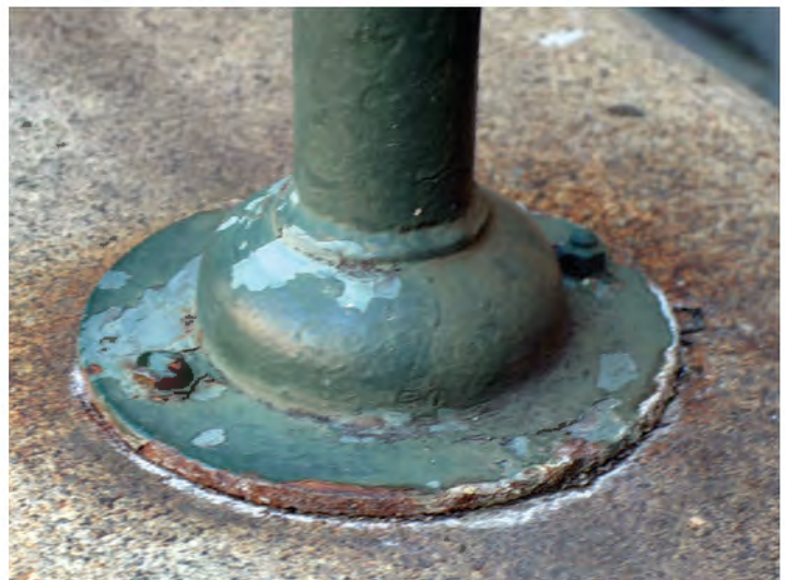
FIGURE 32: 12th Street Moat Railing Post Showing Paint Failure and Corrosion at the Base, 2012. Photo Courtesy OLBN Inc.
