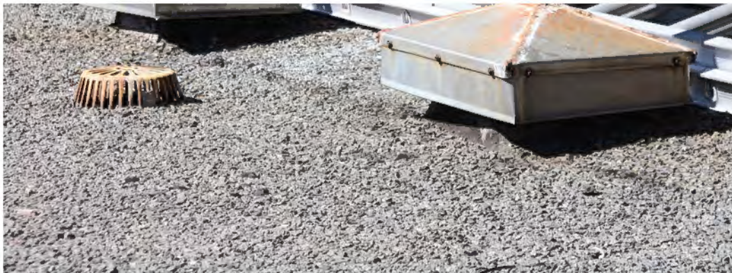
FIGURE 54: There Are Many Roof Penetrations Throughout The Built Up Roof Area, 2012. Photo Courtesy OLBN Inc..
