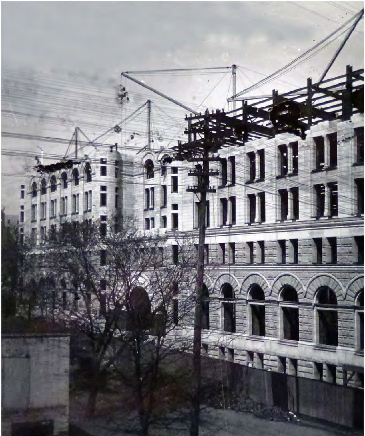
FIGURE 92: Post Office under construction; structural skeleton can be seen behind stone façade. Image Courtesy of the National Archives and Record Administration, Cartographic and Architectural Records, College Park, MD, Record Group 121
