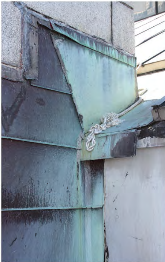
FIGURE 40: Copper Flashing against Clock Tower Wall, 2012. Some of the copper flashing folds and seams have been sealed with a bituminous coating, indicating the presence of leaks. Photo Courtesy OLBN Inc.
