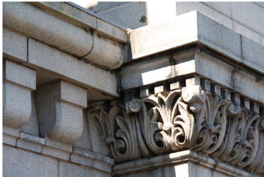
FIGURE 43: Detail of the Clock Tower Cornice /Belt Course, 2012. Photo Courtesy OLBN Inc.
