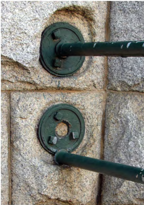
FIGURE 33: 12th Street Broken Moat Railing, 2012. Photo Courtesy OLBN Inc.
