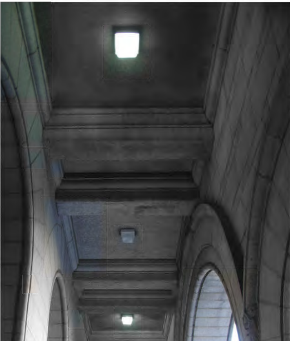
FIGURE 73: 12th Street Portico Ceiling, 2012. Photo Courtesy OLBN Inc.
