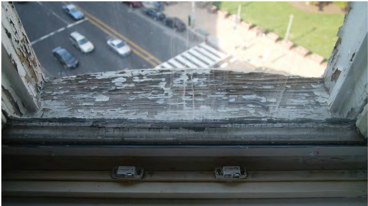
FIGURE 56: Paint Is Almost Gone at the Sill and Lower Section of the Jamb, 2012. Photo Courtesy OLBN Inc..
