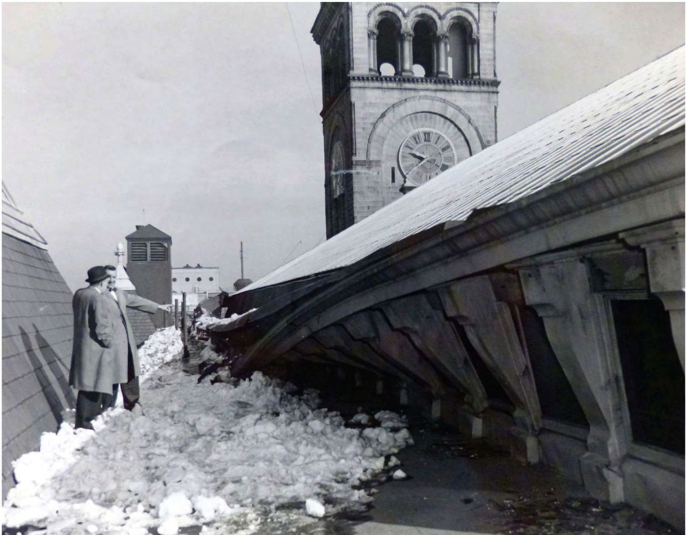
FIGURE 32: Undated photograph of men inspecting roof, showing deteriorated condition of skylight roof clerestory. Image Courtesy of GSA-NCR Technical Resource Center, Reports and Photographs
