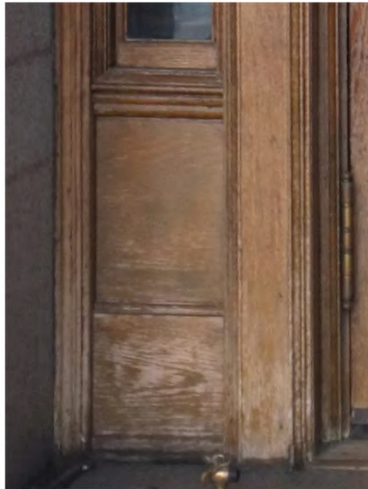
FIGURE 80: Detail of Pennsylvania Avenue NW Door Sidelight Sill, 2012. Photo Courtesy OLBN Inc.
