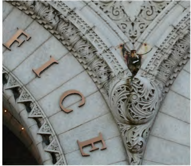
FIGURE 7: Pennsylvania Avenue Portico Rust Staining, September 2012. Photo Courtesy OLBN Inc.
