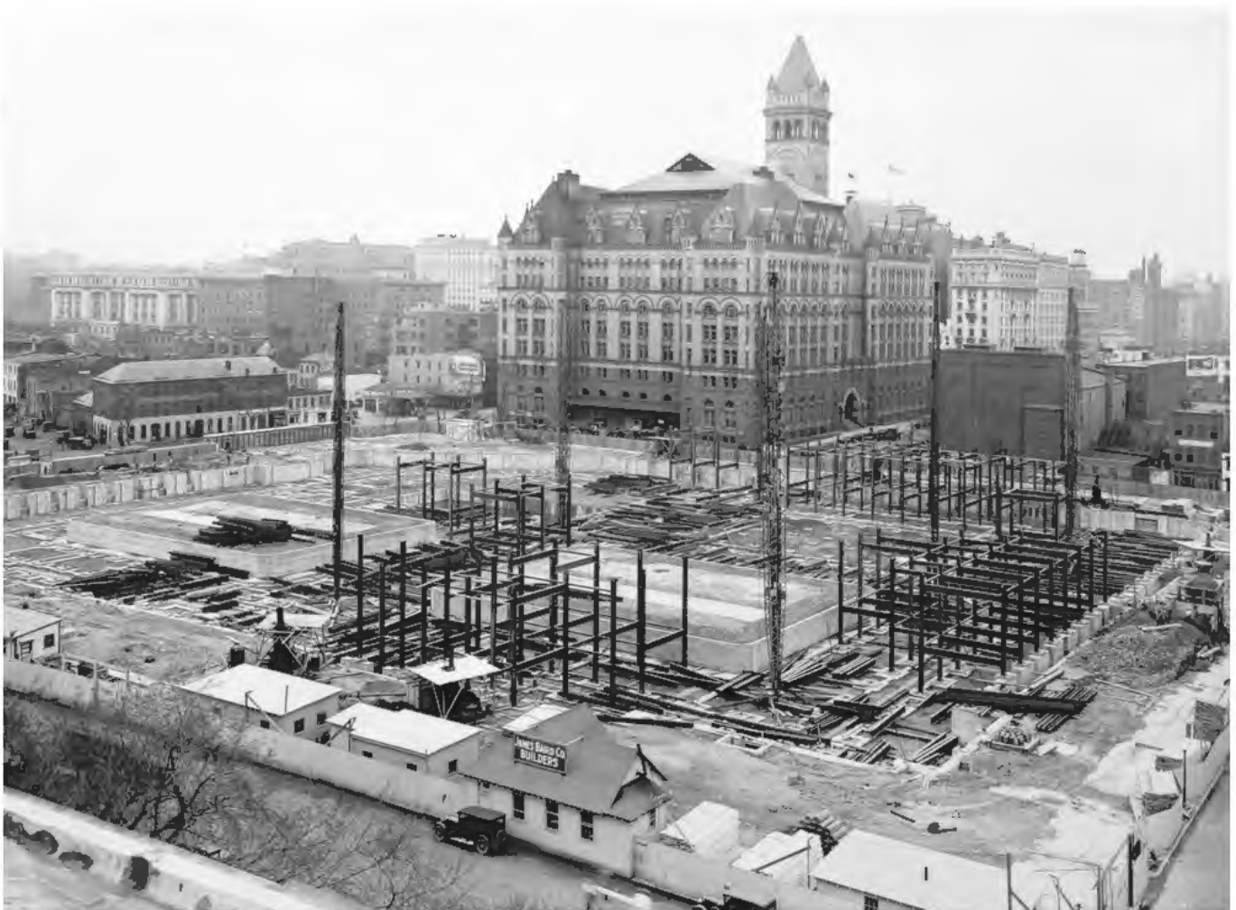
FIGURE 27: 1929 Photograph of IRS Building under construction. Image Courtesy of the Library of Congress, Prints and Photographs Division, HABS Collection
