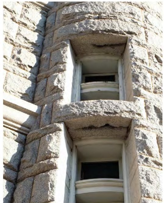
FIGURE 5: Pennsylvania Avenue West Corner Turret Staining and Wash Streaks, September 2012. Photo Courtesy OLBN Inc.
