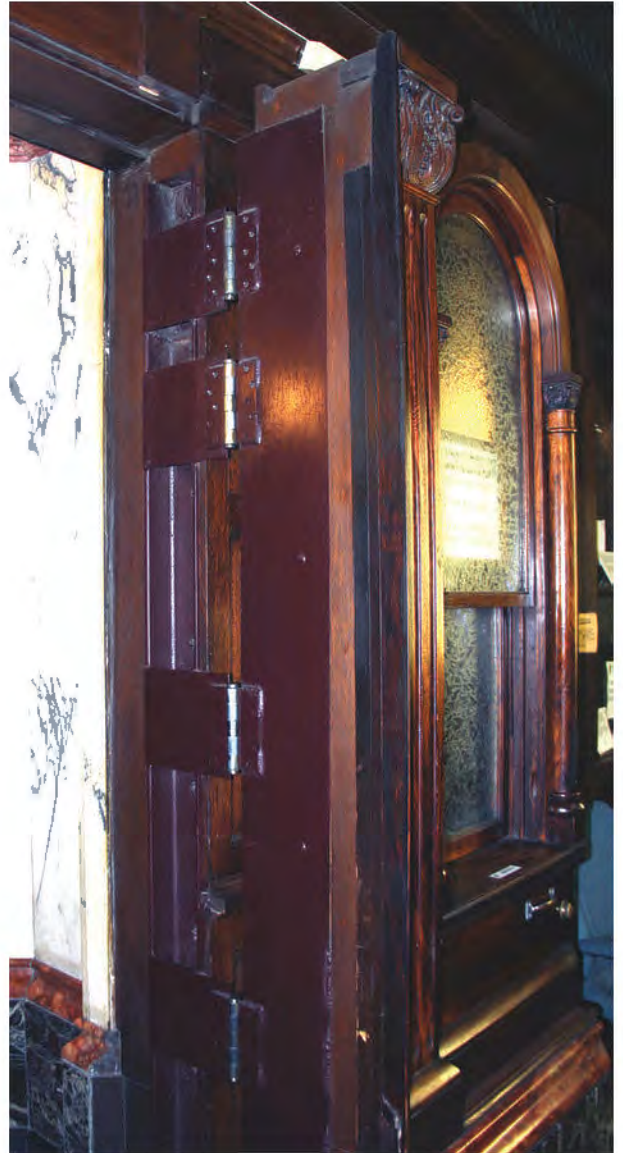
FIGURE 66: Mahogany Feature Wall Showing Hinges Installed in 1979, When a Section of the Door Was Converted into a Door, 2012. Photos Courtesy OLBN Inc..
