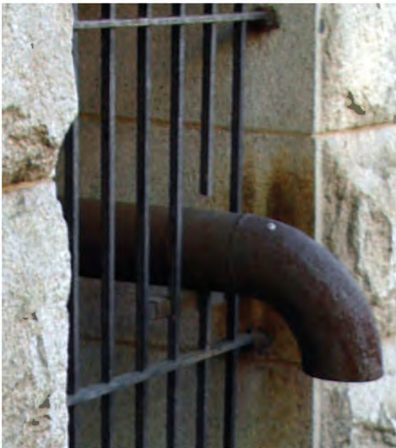
FIGURE 31: Pennsylvania Avenue Window Guard. Its Anchoring Points Are Corroded, 2012. Photo Courtesy OLBN Inc.
