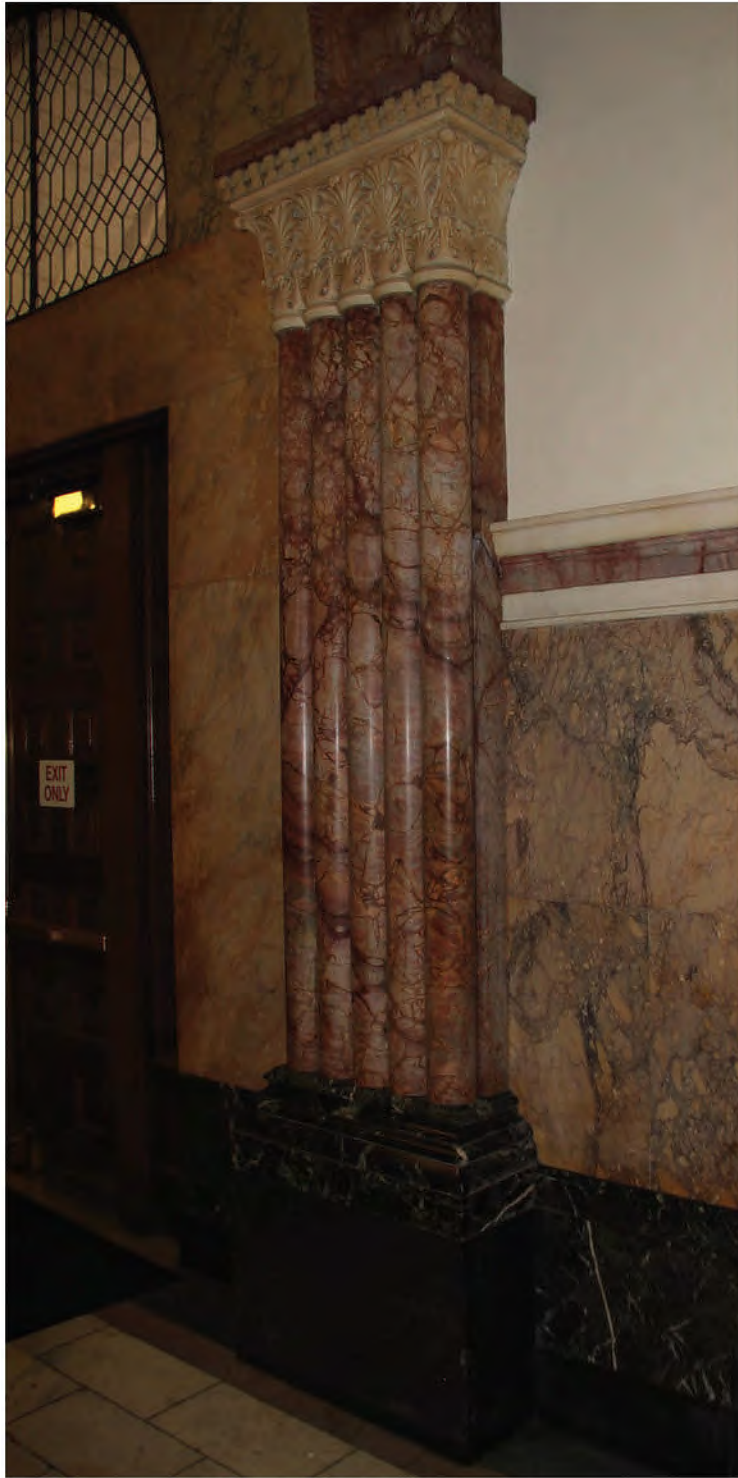
FIGURE 85: Pennsylvania Avenue NW Pilaster, 2012. Photos Courtesy OLBN Inc.
