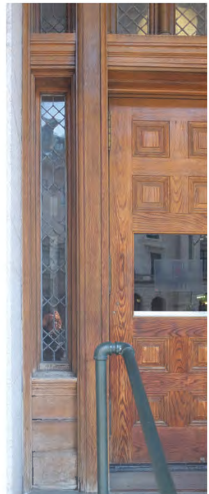
FIGURE 61: Exterior Door Sidelight, 2012. There is damage and deterioration below the glass panels, where water can rise through the end grain of the wood. Photo Courtesy OLBN Inc..
