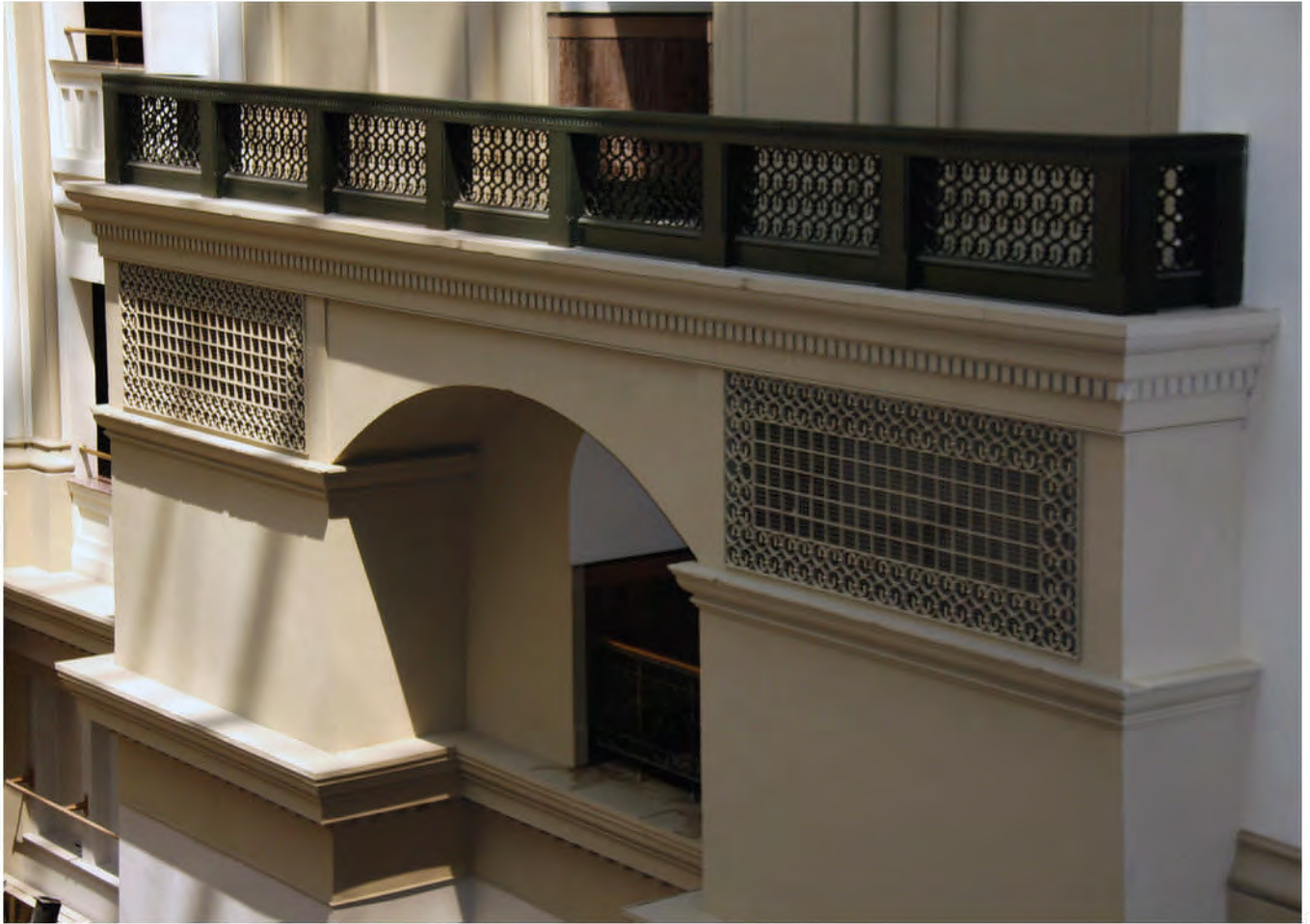
FIGURE 1: Interior View of Third Floor Balcony, Old Post Office, November 2012. Image courtesy OLBN Inc.
