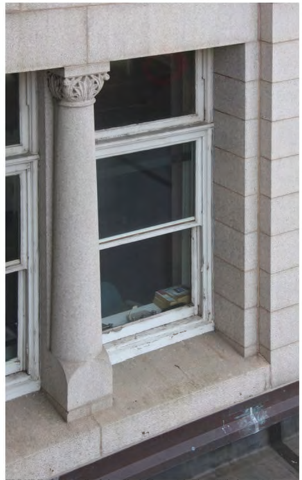
FIGURE 38: Detail of the Clock Tower 3rd Floor Window, 2012. Photo Courtesy OLBN Inc.
