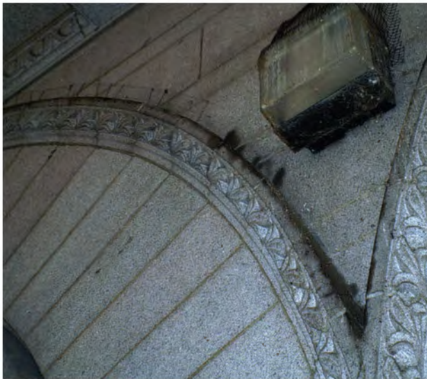
FIGURE 9: Pennsylvania Avenue Portico Pigeon Guano, September 2012. Photo Courtesy OLBN Inc.
