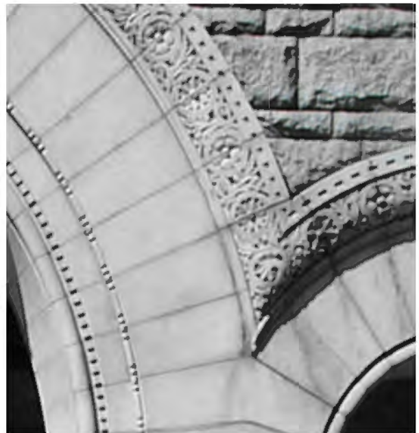
FIGURE 65: 11th Street Archway moulding Detail, 2012. Photo Courtesy OLBN Inc.
