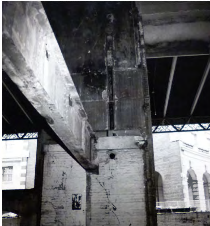
FIGURE 98: Washington D.C. Post Office, Condition of Basement Prior to 1979 Renovation. Image Courtesy of GSA-NCR Technical Resource Center.
