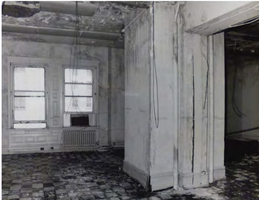
FIGURE 97: Washington D.C. Post Office, Condition of Office Space Prior to 1979 Renovation. Image Courtesy of GSA-NCR Technical Resource Center.
