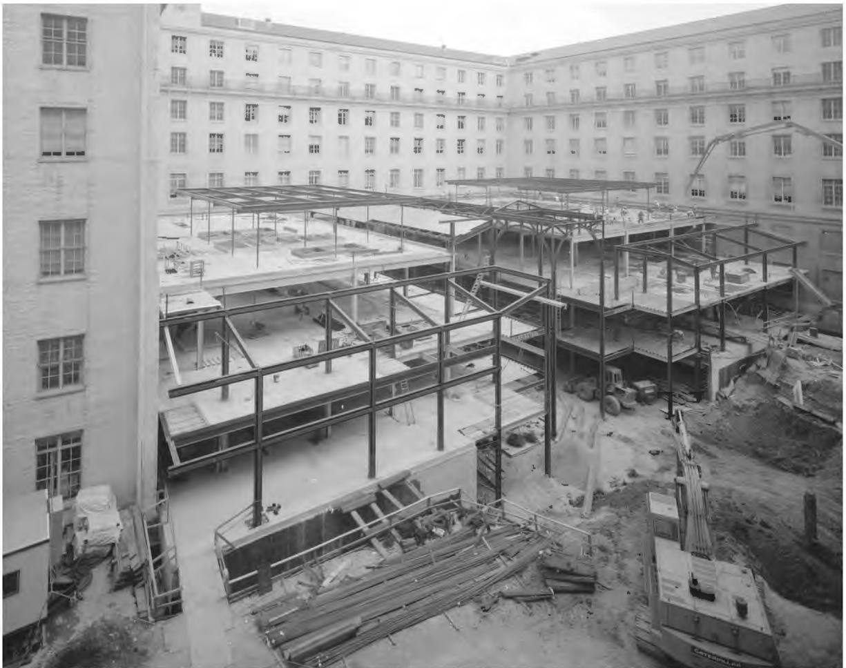
FIGURE 42: The Atrium under construction, 1991. Image Courtesy of the Library of Congress, Prints and Photographs Division, HABS Collection
