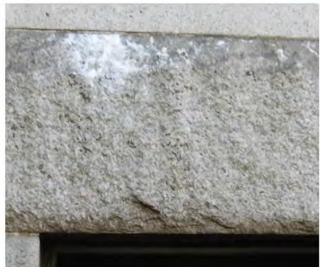
FIGURE 8: Pennsylvania Avenue Wall Mineral Deposits, September 2012. Photo Courtesy OLBN Inc.
