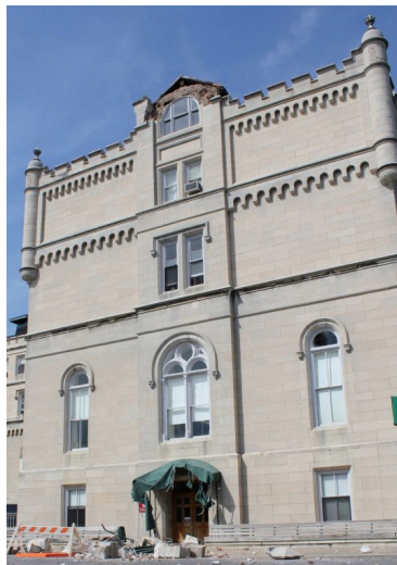
Collapsed gable, Sherman North
