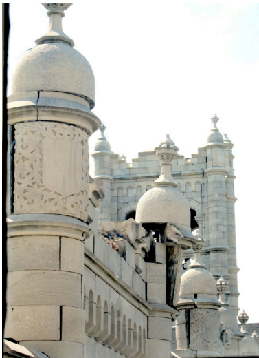
Unstable parapets, Sherman Annex
