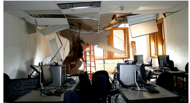
Damage under clock tower, Sherman South
